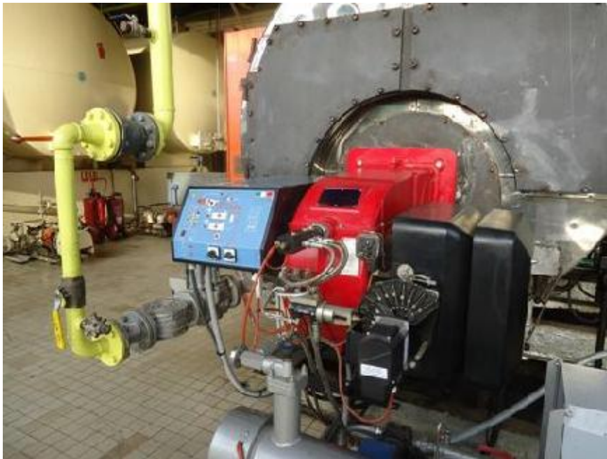
Boiler Refurbishment / Natural Gas Burner
